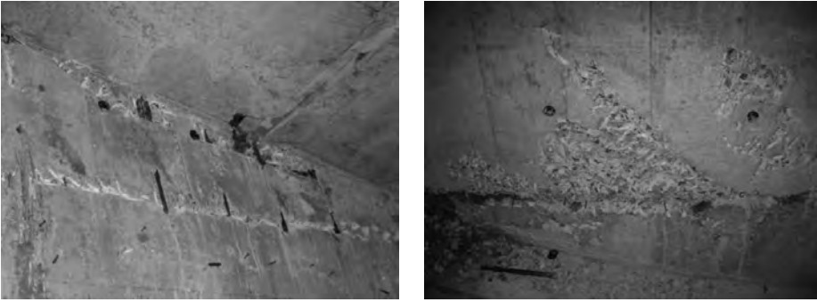
Fig. 7.7: Spalling and delamination in the existing structure
