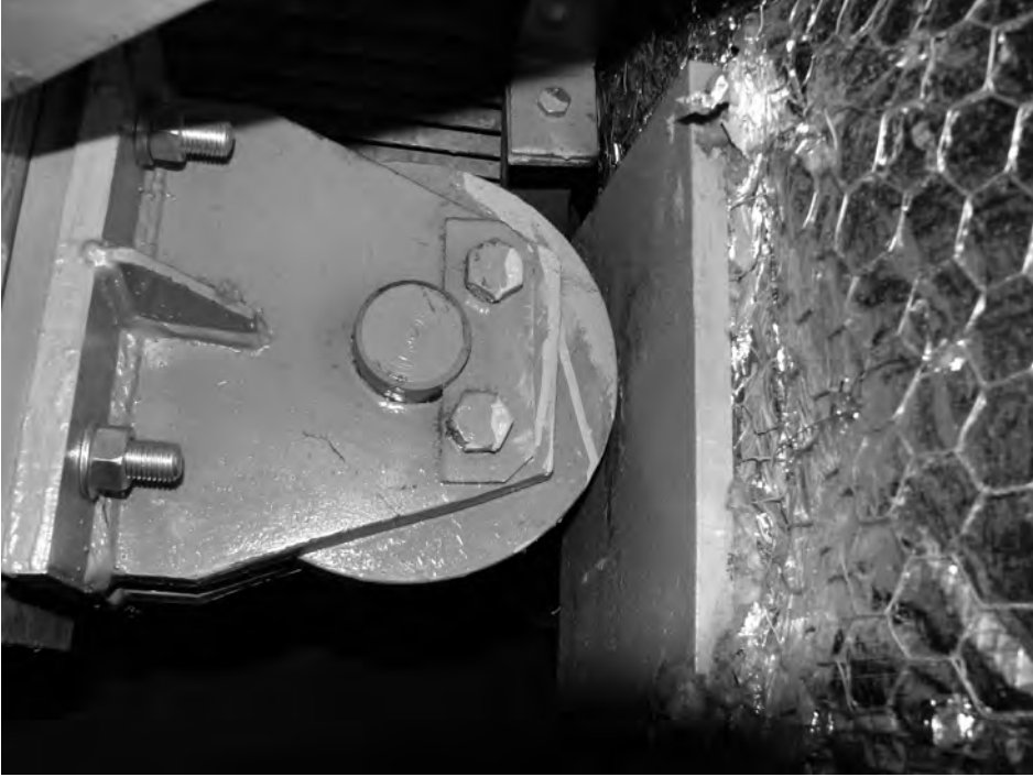
Fig. 6.13: A roller stabilizing the smoke conduit in the level of intermediate platform
