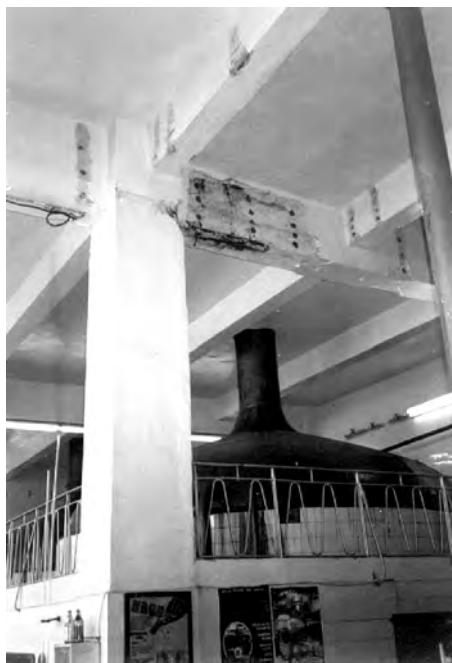
Fig. 5.6: Damage of main beams
