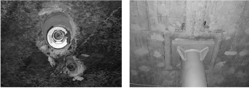
Fig. 4.25: Embedded and injected anchor head next to an unfinished hole and concrete surface after strengthening
