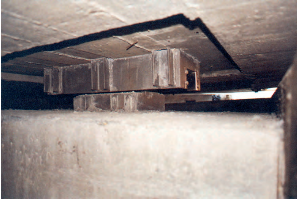
Fig. 2.6: Fixed bearings at the abutments were replaced by the unidirectional sliding bearings
