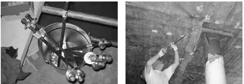
Fig. 4.24: Adjusted HZA-P anchors to the individual hole depth and installing in the hole
