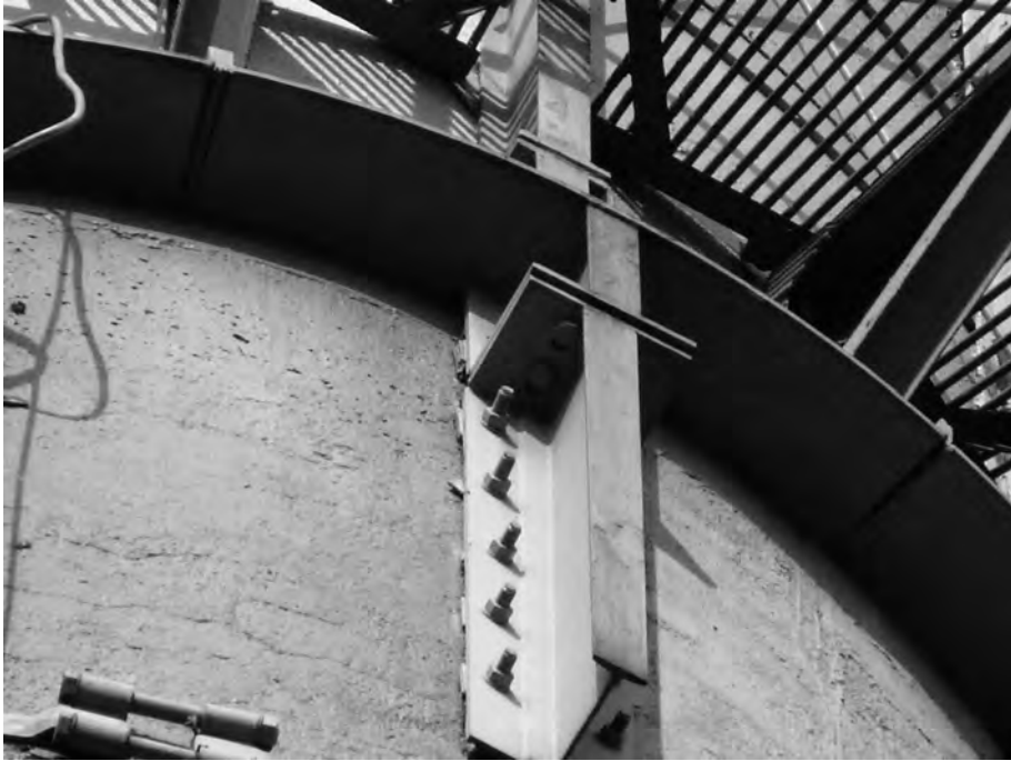
Fig. 6.7: The detail of anchoring the steel members to the outer RC jacket
