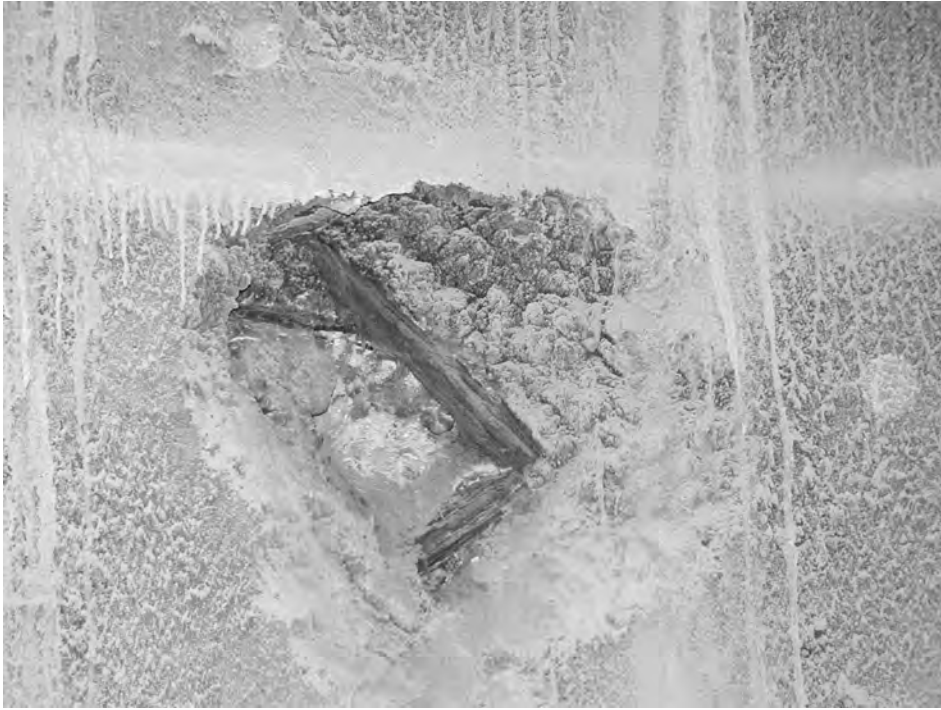
Fig. 6.15: Shaft's inner surface; an example of uncovered and corroded reinforcement
