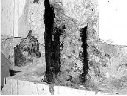
Fig. 5.7: Damage of columns
