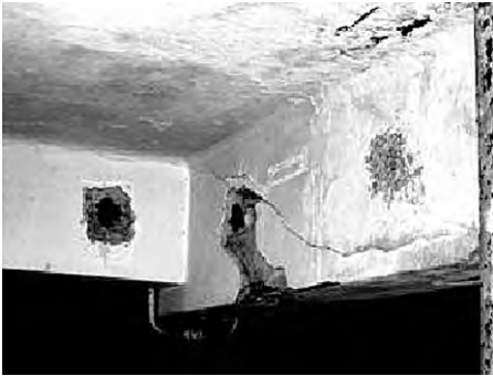
Fig. 5.8: Inclined cracks at main beams
