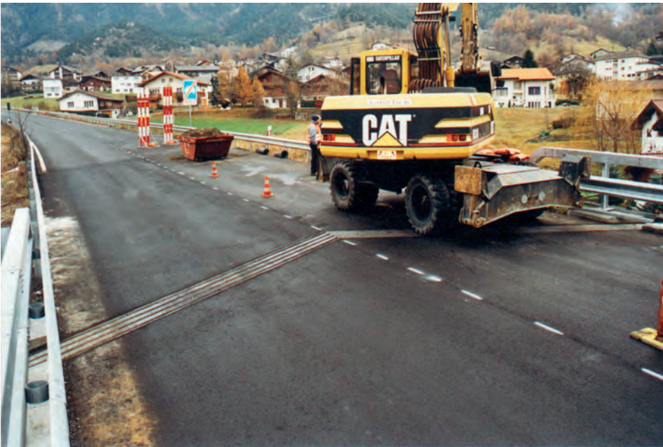
Fig. 2.9: Joints at the bridge ends have been replaced by larger ones with V-shape [1]
