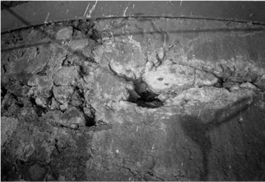
Fig. 6.3: An example of outer jacket damage
