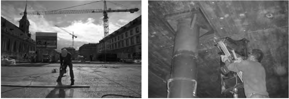
Fig. 4.22: Drilling for anchoring of upper tensile reinforcement and for punching shear reinforcement
