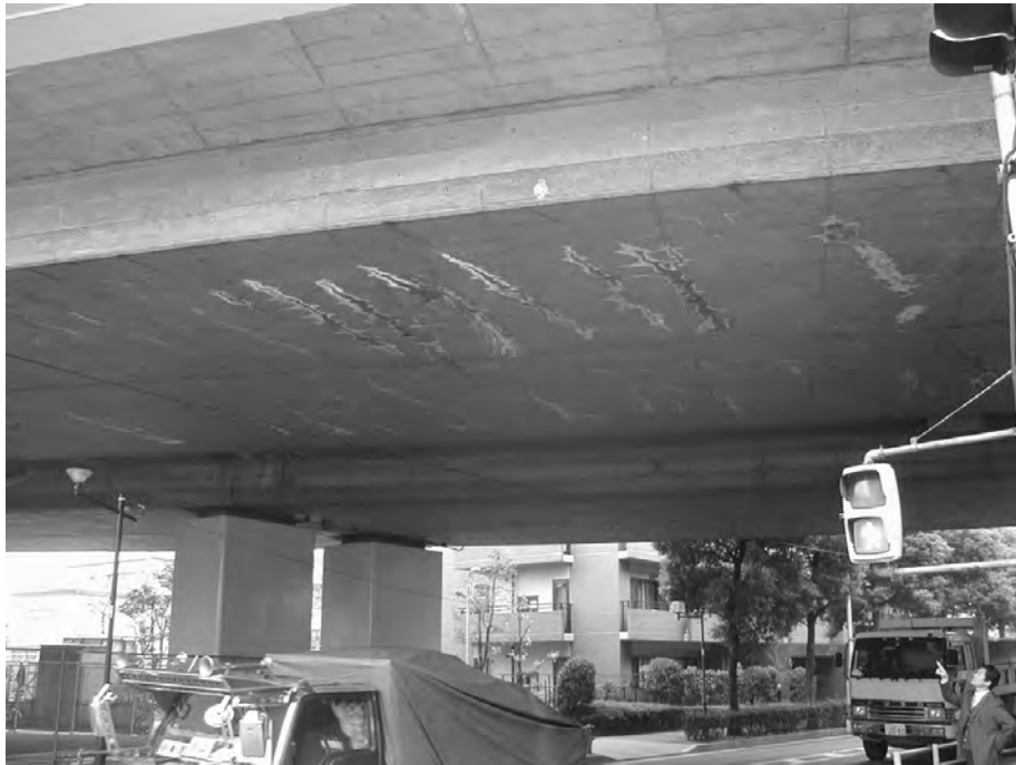
Fig. 3.2: State of damages
