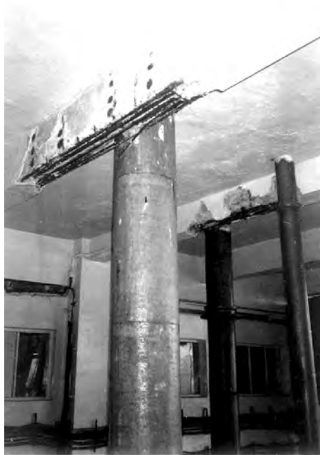
Fig. 5.5: Damage of secondary beams
