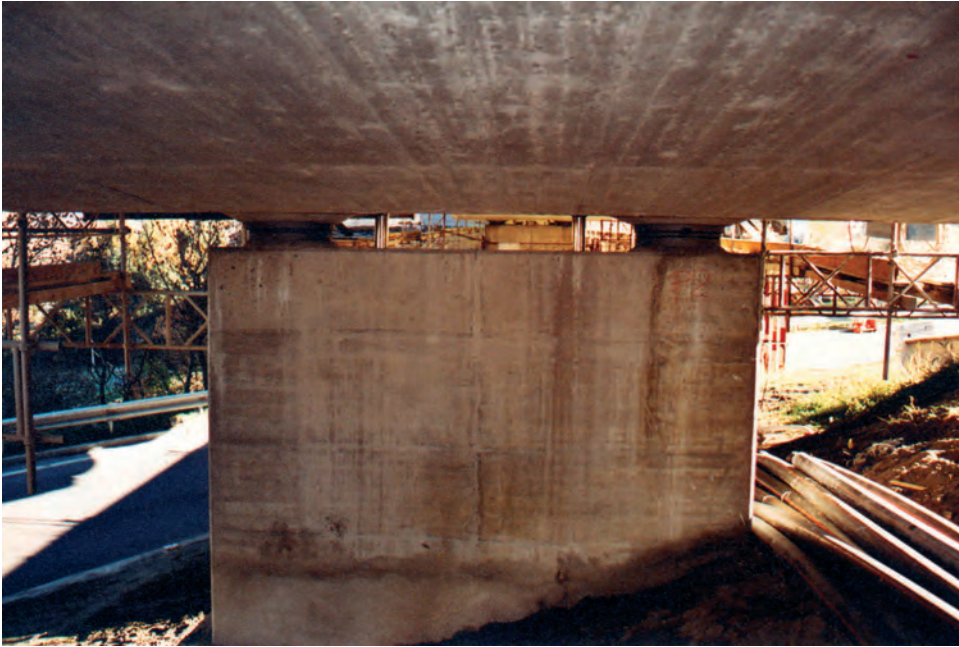
Fig. 2.5: Rustproof steel bars D = 80 mm on the pier heads [1]
