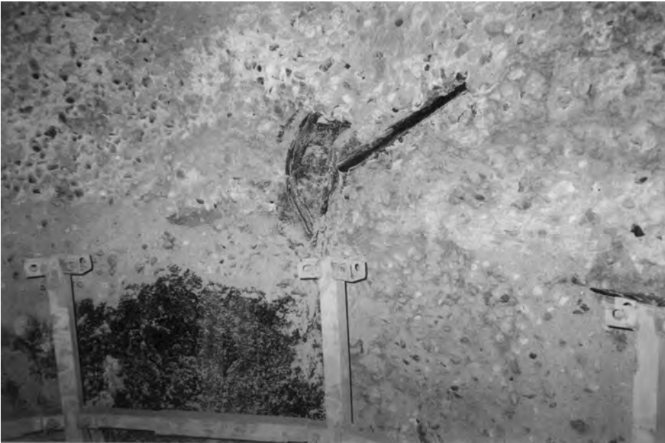
Fig. 6.14: An example of concrete surface damages on the inner surface of the carrying shaft
