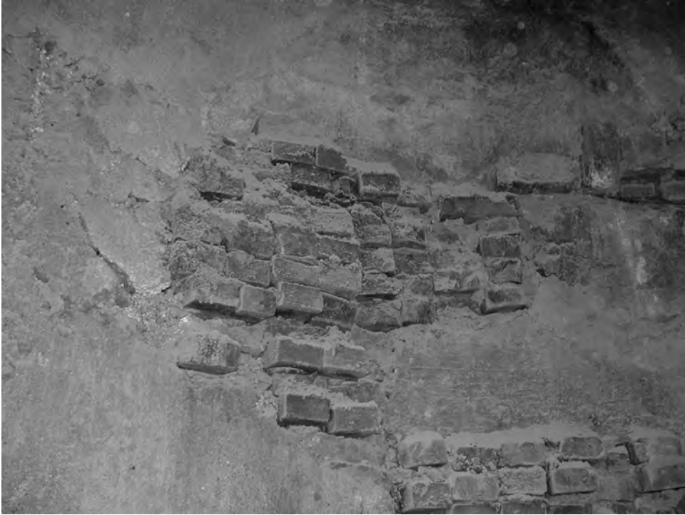
Fig. 6.16: Shaft's inner surface faults; visible void fillings with ceramic brick (outside masked with cement plaster)
