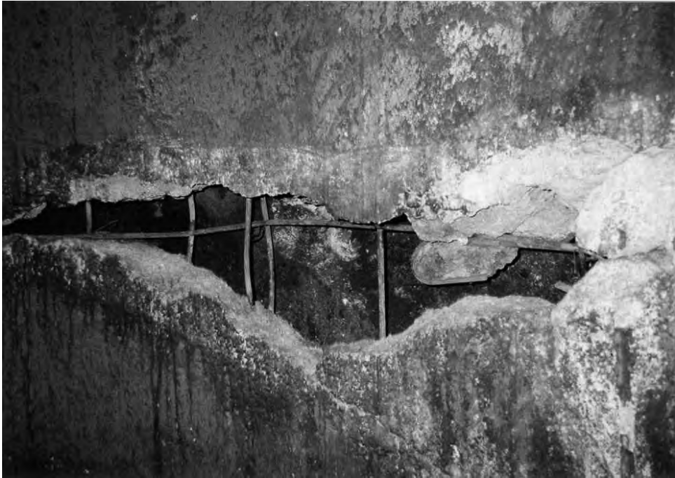
Fig. 6.4: An example of inner jacket damage
